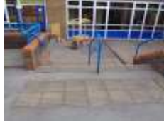
Below picture – nosings needed here.
